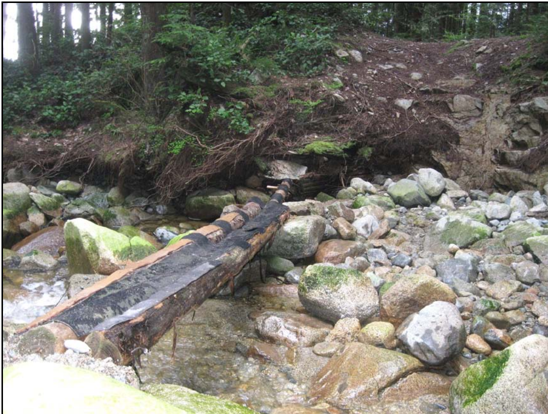
In Pinecone Burke Park, protected in 1995, a temporary log crossing built by volunteers provides low-water passage over Pritchett Creek on the popular Woodland Walk trail. With adequate funding, BC Parks could construct a proper footbridge. Ian McArthur photo.
